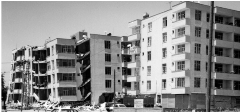
Figure 4. Aspect of the damages on modern constructions at the eastern sector of Ceyhan.
