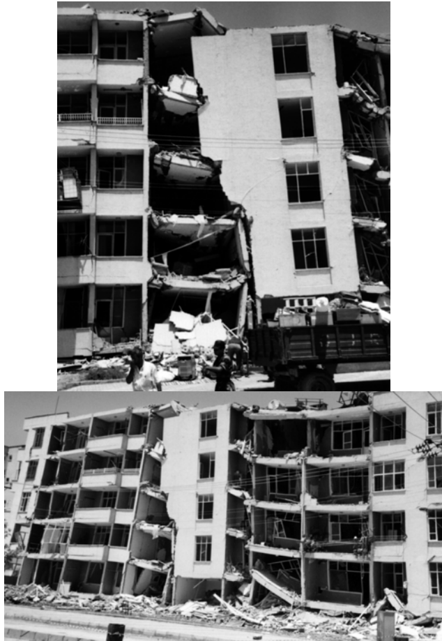
Figure 7. Aspects of a modern multi-story construction of NE-SW orientation, which collapsed totally.
